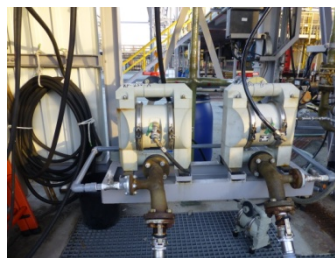
Pumps with flush lines
